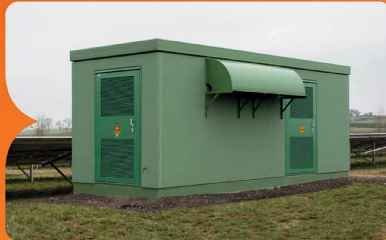
Inverter / transformer units
